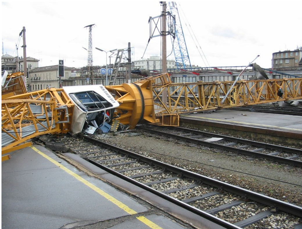
Gale “Emma” – overturned crane, Vienna, 2008
